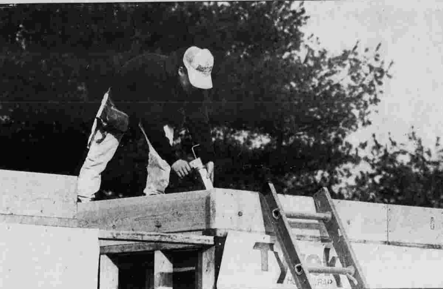
FLOOR WORK — Rick Cramer of Coventry, an employee of R.B.M. Building of Willington, glues flooring for the Ansaldo Apartments at the corner of Wetherell and Bidwell streets Monday.
